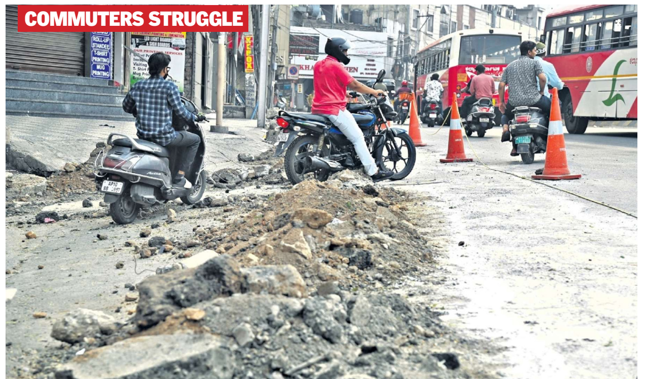
Commuters struggle to navigate a badly damaged road at Lakdikapul on Sunday as delayed construction work and poor maintenance create hardships for motorists, raising concerns over traffic safety and civic neglect.
